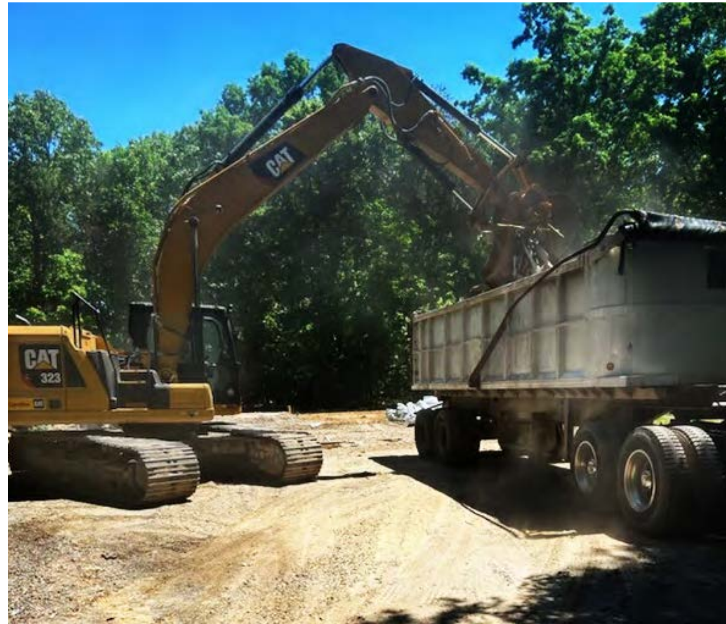
↑ Since beginning geological activities at Carolina Lithium, we have worked closely with S.C. Lovelace and Sons, a local contractor experienced in the mining industry. Lovelace performs a range of earthworks, including reclamation activities when homes are purchased and no longer needed on the project site.
